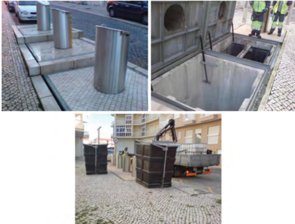
Figure 1: Represented the Underground Waste Containers.
