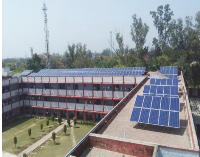
Figure 1: Rooftop solar plates for electricity generation in education institutions[5].
