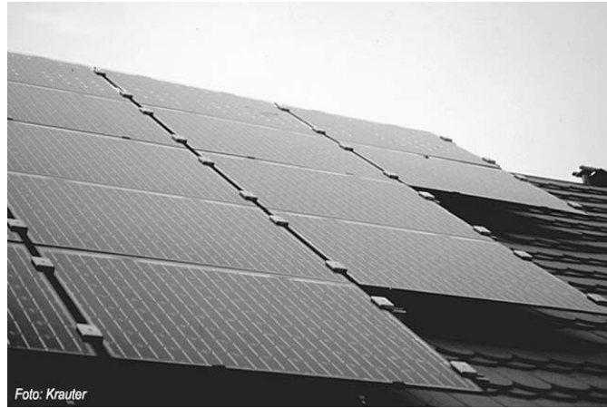
Figure 13.9: The Roof-mounted PV generator with frameless modules and fixture compounds.
